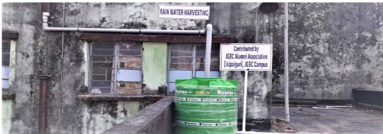
Figure: Sample of rainwater harvesting
